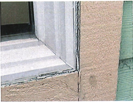
Deteriorating caulking around several exterior window trims.
