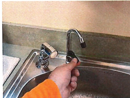
Filtered faucet in kitchen did not operate
