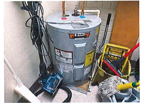
FYI - Water heater in mechanical closet near kitchen in hallway
