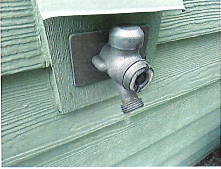
No handle on faucet on South side
