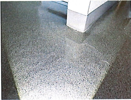
Leak underneath dishwasher
