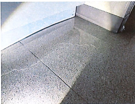
Leak underneath dishwasher
