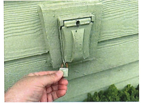
FYI - Several exterior outlets covers are padlocked shut.
