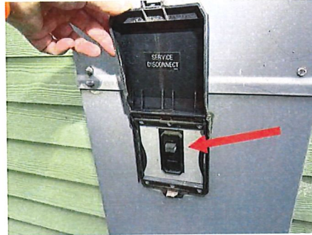
FYI - Main electric service disconnect breaker panel & meter box on West side in alley
