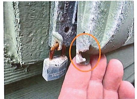
Some exterior outlets are not locked - have damaged covers that will not lock
