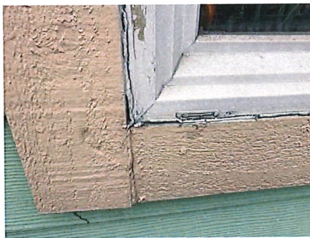
Deteriorating caulking around several exterior window trims.
