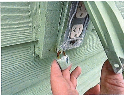
Some exterior outlets are not locked - have damaged covers that will not lock
