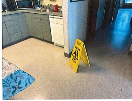
Leak underneath dishwasher
