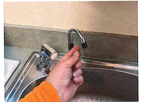
Filtered faucet in kitchen did not operate
