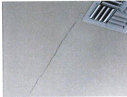
Crack in ceiling drywall over secured storage room area on East side main room
