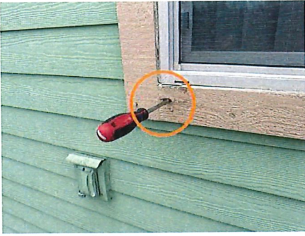
Wood rot on window trim - SW side
