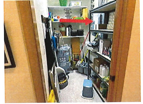
FYI - Electric subpanel in mechanical closet near kitchen hallway
