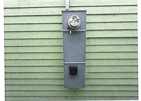
FYI - Main electric service disconnect breaker panel & meter box on West side in alley
