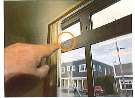
Window crank handle missing on window in NE office
