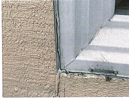
Deteriorating caulking around several exterior window trims.
