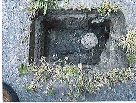
FYI - Water meter in sidewalk by front entry steps
