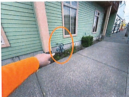
Natural gas meter & main shut off on front of building
