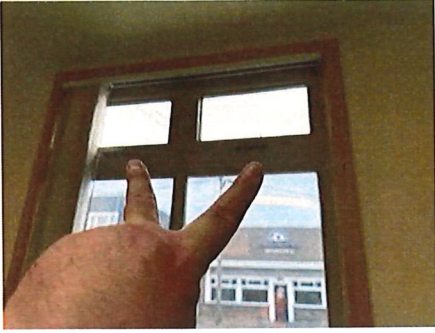
Window crank handle missing on window in NE office
