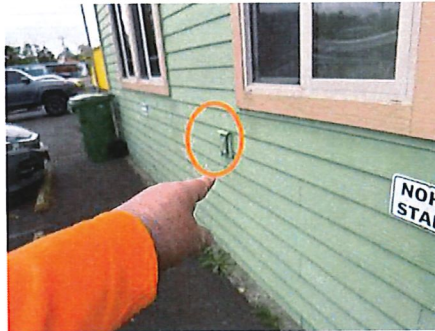
Some exterior outlets are not locked - have damaged covers that will not lock
