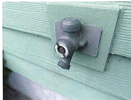
No handle on faucet on front sidewalk
