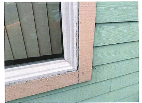
Deteriorating caulking around several exterior window trims.
