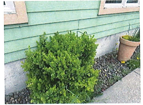
Some vegetation contacting building - should be trimmed to at least >12" away from structure.
