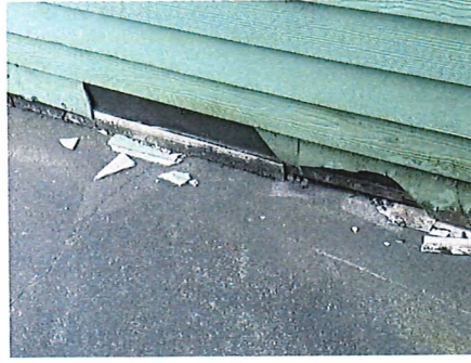
Some damage to lowest course of siding at west side alley.
