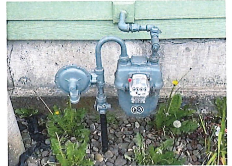
Natural gas meter & main shut off on front of building
