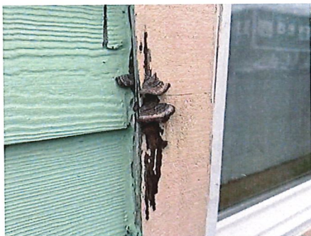
Wood rot on window trim - Front side 4th window from left as facing
