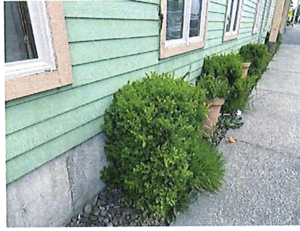
Some vegetation contacting building - should be trimmed to at least >12" away from structure.
