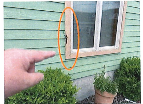
Wood rot on window trim - Front side 4th window from left as facing
