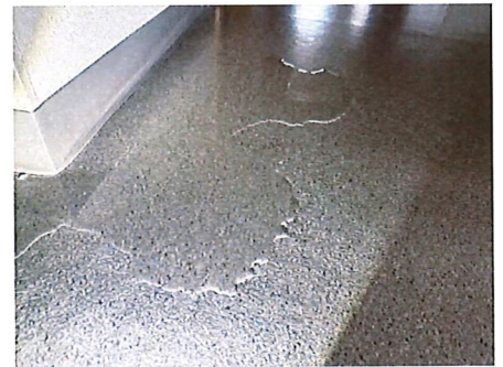
Leak underneath dishwasher
