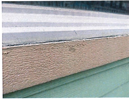
Deteriorating caulking around several exterior window trims.
