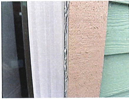
Deteriorating caulking around several exterior window trims.
