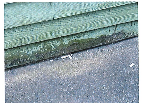
Some damage to lowest course of siding at west side alley.
