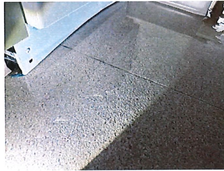
Leak underneath dishwasher
