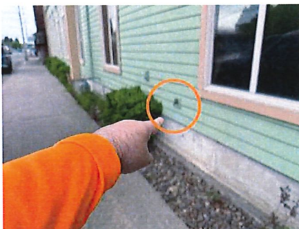
No handle on faucet on front sidewalk
