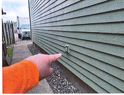
Some exterior outlets are not locked
