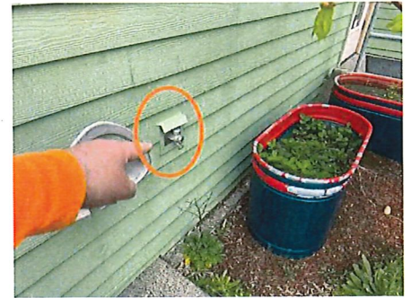
No handle on faucet on South side
