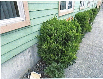
Some vegetation contacting building - should be trimmed to at least >12" away from structure.
