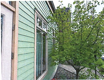
Some vegetation contacting building - should be trimmed to at least >12" away from structure.
