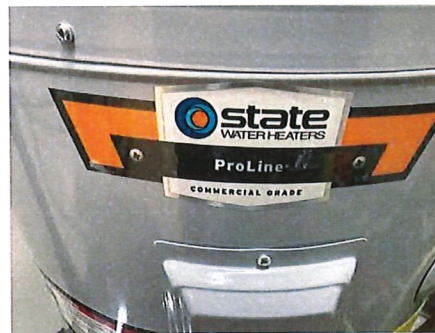
FYI - Water heater in mechanical closet near kitchen in hallway
