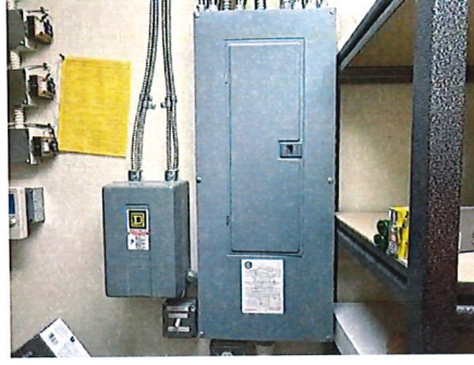
FYI - Electric subpanel in mechanical closet near kitchen hallway
