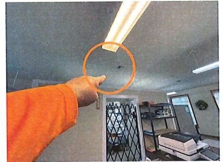
Crack in ceiling drywall over secured storage room area on East side main room
