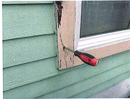
Wood rot on window trim - Front side 4th window from left as facing
