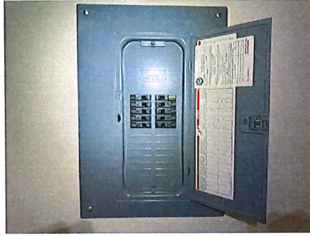
FYI - 2nd subpanel in main room on South side
