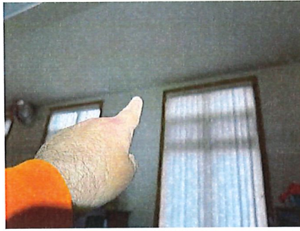
Crack in drywall over windows on SE area of main room
