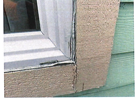
Deteriorating caulking around several exterior window trims.
