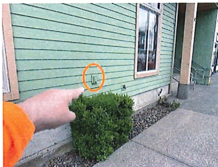
FYI - Several exterior outlets covers are padlocked shut.
